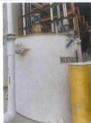
Bể Trung hòa pH
